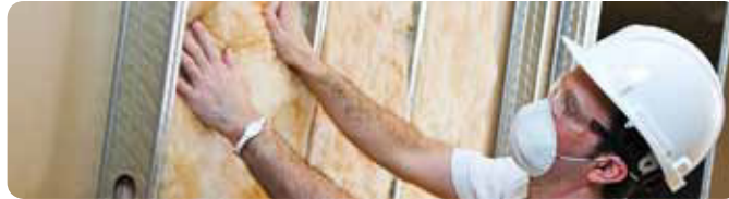
CertaPro™ Commercial Insulation
